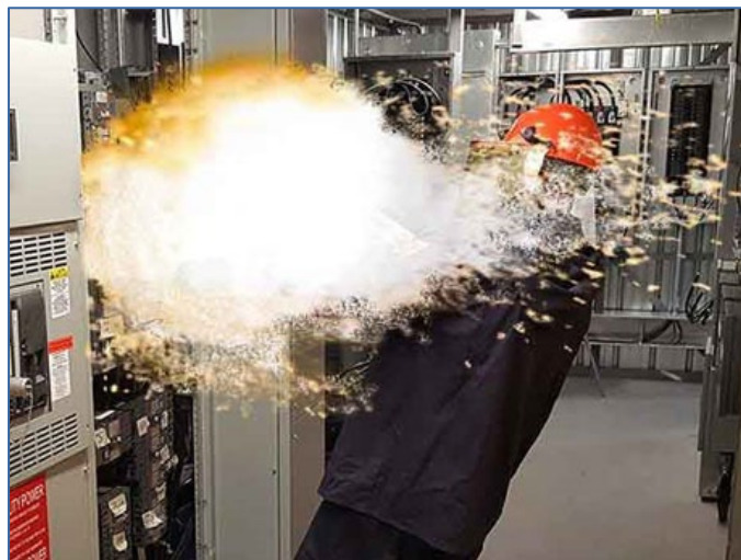
Electrical arc flash
