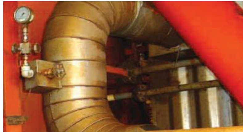
Images: Corrosion under insulation – Courtesy Health and Safety Executive 2006
