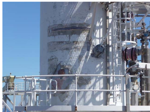
Figure 2 - Damage to the PFP on the Debutaniser Column
