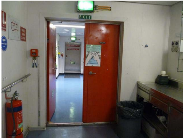
Figure 9 - A60 Fire Door to the Mess Room (TR)
