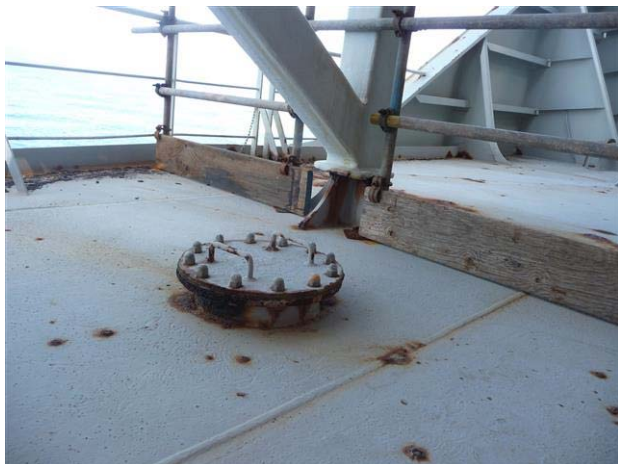
Figure 7 - Corrosion at Deck Penetration
