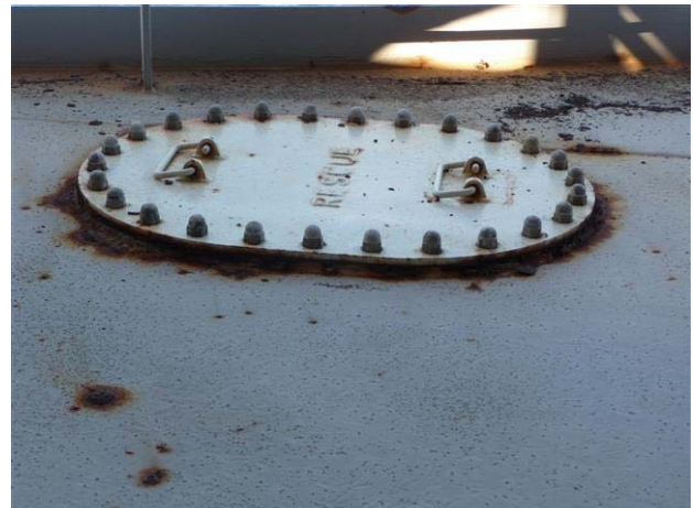
Figure 6 – Corrosion at Deck Penetration
