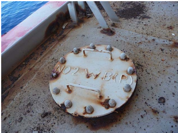
Figure 5 - Corrosion on the #2 Water Ballast Tank
