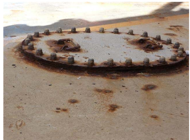
Figure 8 - Corrosion at Deck Penetration
