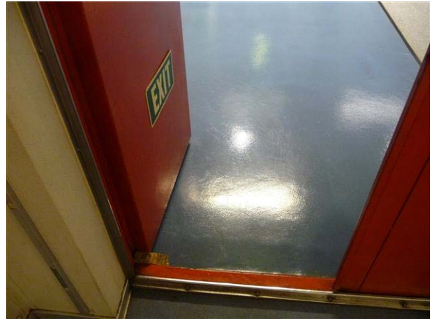
Figure 10 - A60 Fire Door to the Mess Room (TR) Showing Wedge
