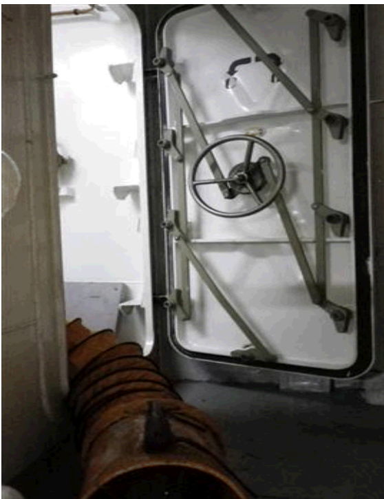
Photo 1 – Water tight door to High Precision Acoustic Positioning System space, marked “To be kept closed at sea” left open and blocked with ventilation trunking. The facility was in Dynamic Position mode close to a petroleum production platform.
