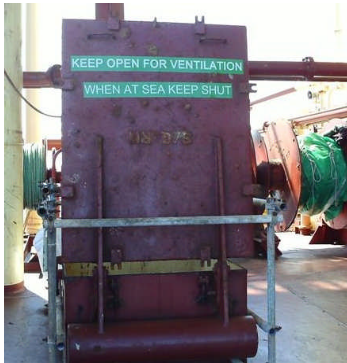
Photo 2 – A large hatch on an FPSO was left open while the FPSO was connected to a buoy. The hatch leads to lower machinery spaces. The hatch is clearly marked “When at sea keep shut”.
