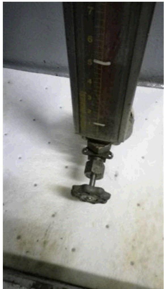
The picture above shows a liquid storage tank sight glass fitted with screw down valves instead of a spring loaded valve.
