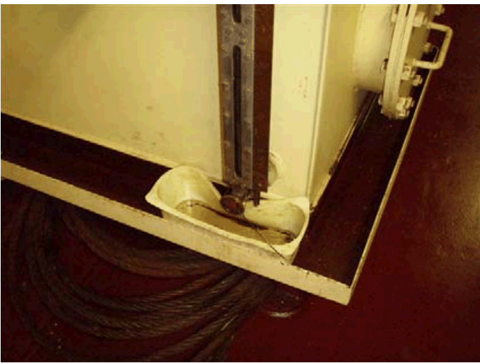
The picture above shows a sight glass for a lube oil tank in a machinery space. Not only is the valve leaking but it is zip tied in the open position.
