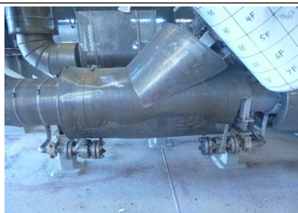
Figure 2 – Debutaniser preheater feed inlet braced to deck SBC
