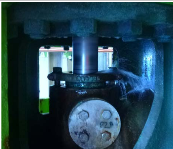
Figure 7 – leaking seawater fire pump B
