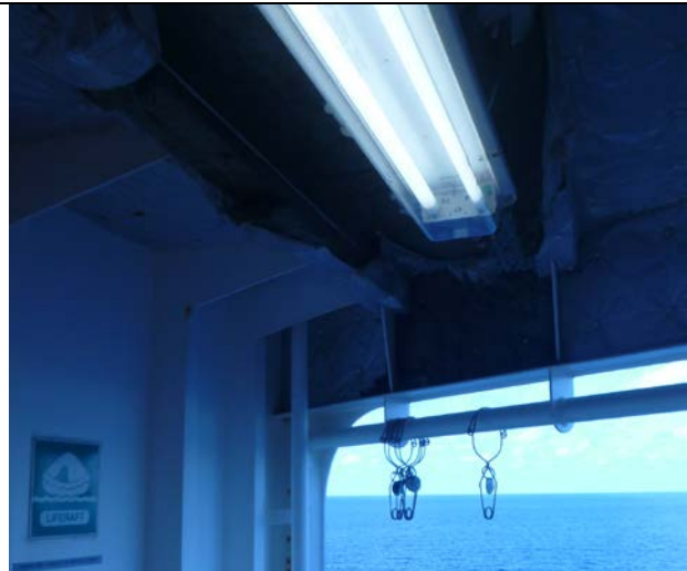
Figure 8 – Damaged fire protection Fwd life raft station
