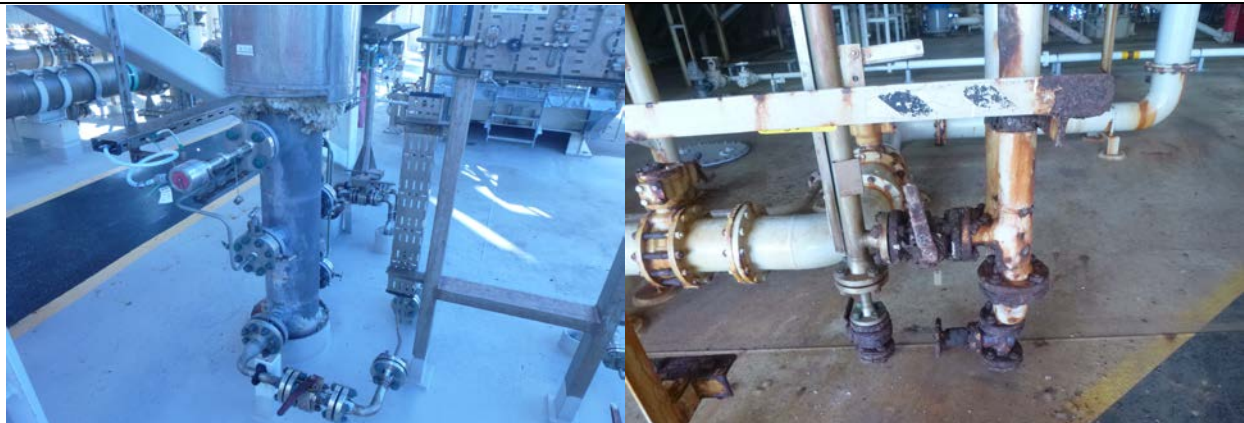
Figure 3 – LPG pump A discharge line insulation Figure 4 – Corroded open drains level gauge
