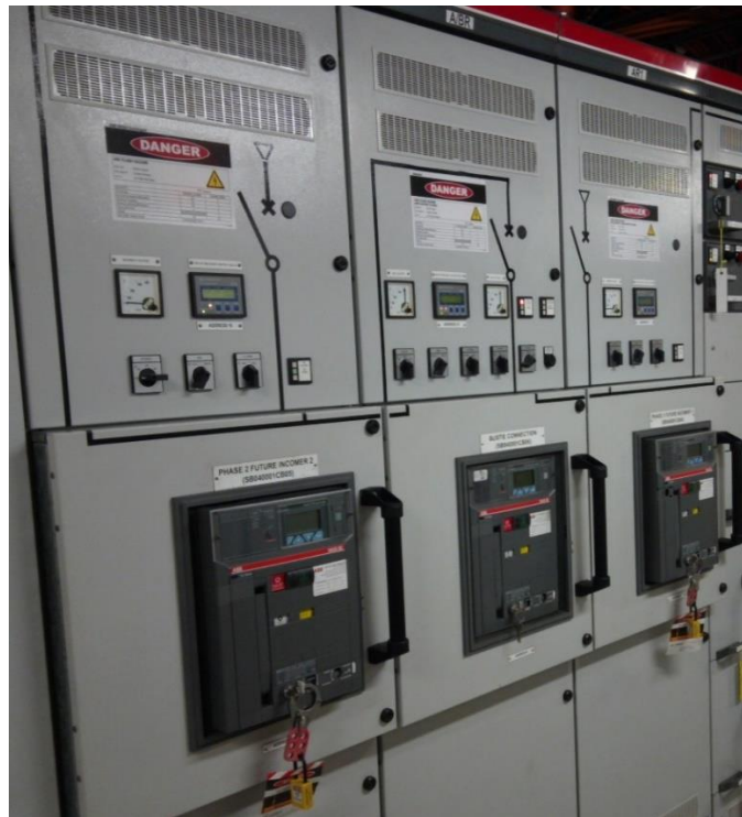
'Danger' arc flash labelling observed on facility low voltage switchboard
