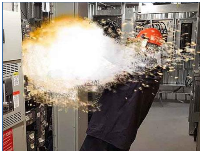
Electrical arc flash
